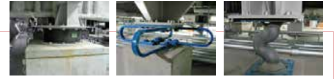
- K computer consists of 864 cabinet racks, at approximately 1,350 kg per cabinet. (In addition, 216 cabinet racks of magnetic disks are installed.)
